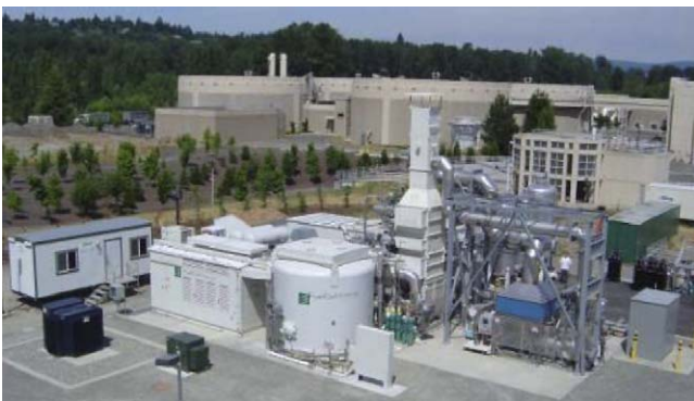
Fig. 10. King county DFC1500 fuel cell power plant: the plant operates on digester gas and on natural gas when digester gas is not available.
